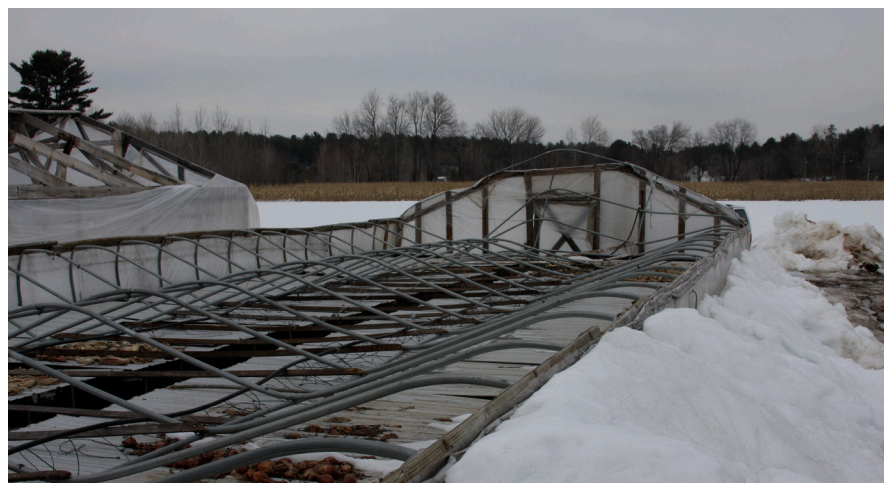
Figure 1. A collapsed double-poly house caused by too heavy of a snow load
