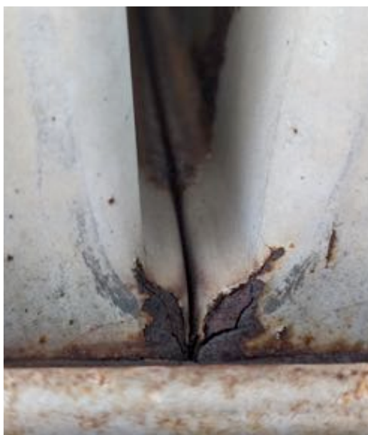
Figure 1. Cracks in the heat exchanger are more easily detected when it is near sunset. (Photo: Brian Whipker)
